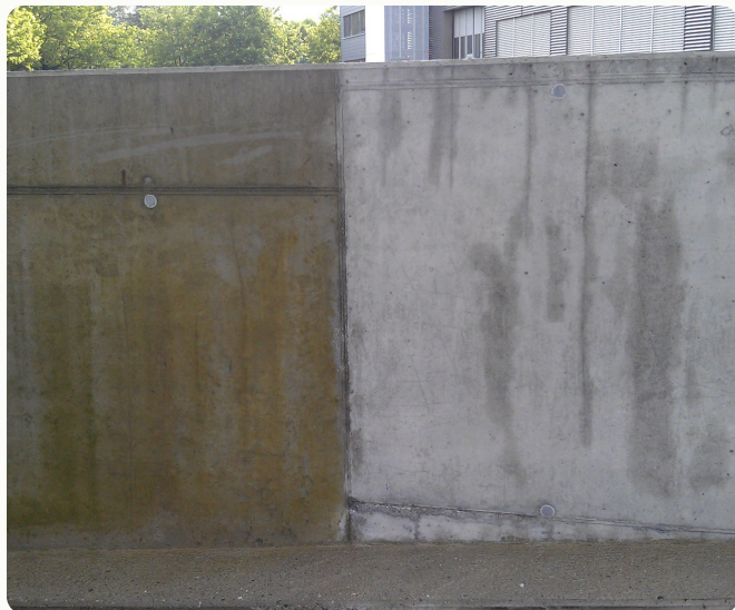
Without protection: dirt, algae, damp patches
